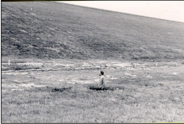
Figure 3-1. Man Standing in Sinkhole
