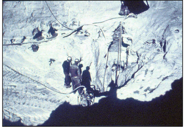
Figure 3-2. Cavern in Foundation Area
