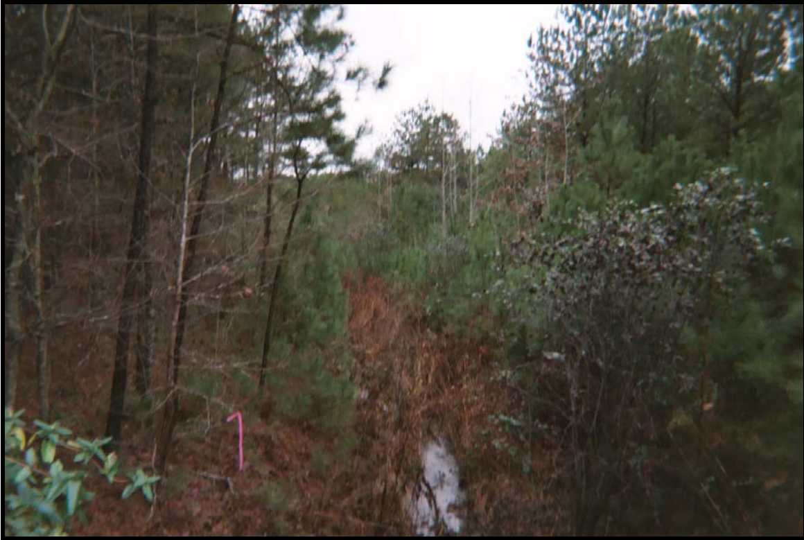
Photograph 1: Landfill No. 3 – Creek channel bordering landfill at a point near Gobbler Road.
