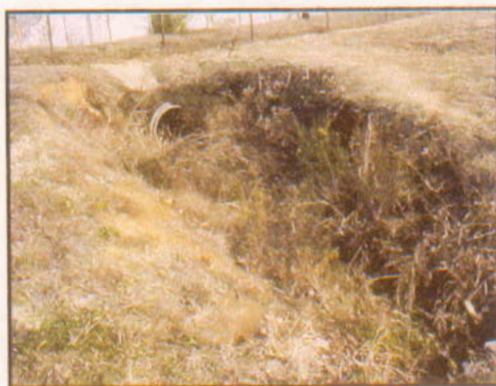
Photograph 2 Outfall at intersection of Mullen and Ball Streets Sample location DDE-SE07
