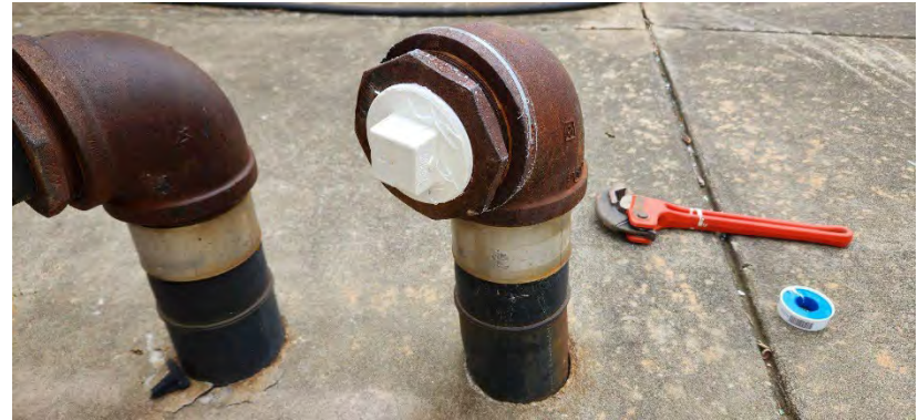
EW-12 Standpipe Permanent Cap
