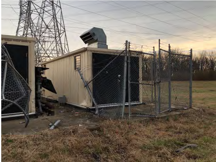
Fence and Gate Damage
