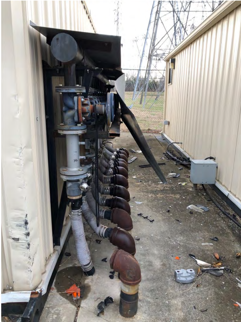
SVE-12 Standpipe and Valve Bank Cover Damage
