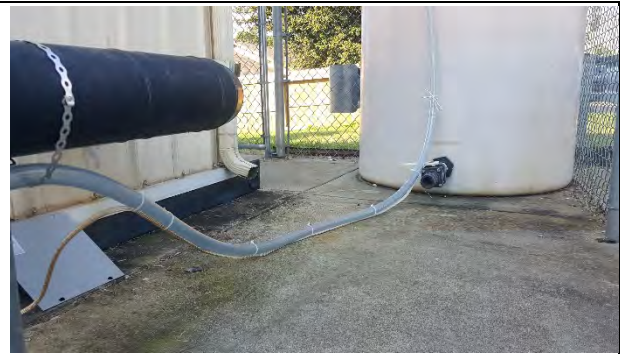
Photograph 14 Condensate line heater tape
