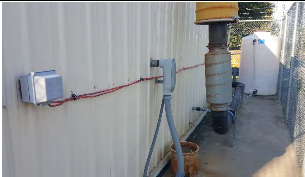
Photograph 15 Heater tape electrical
