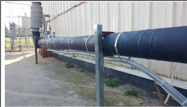
Photograph 13 Condensate line placement
