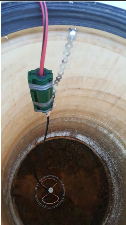
Photograph 17 Submersible tank heater
