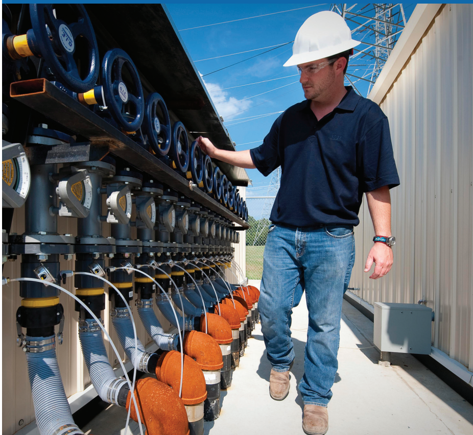
Brad Sperry of HDR, environmental contractors to the Army, monitors the Off-Depot Groundwater air sparge-soil vapor extraction system that is removing contaminants from groundwater west of Dunn Field.
