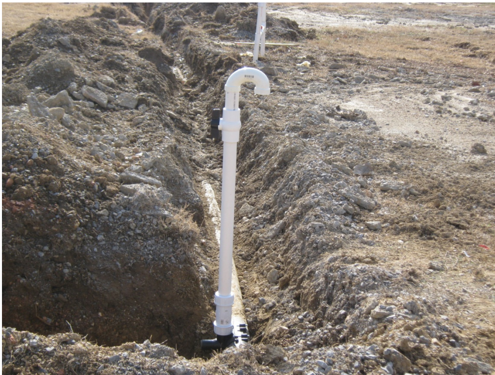
Photograph 6: Vents were installed on SVE-G line to aid condensate removal.
