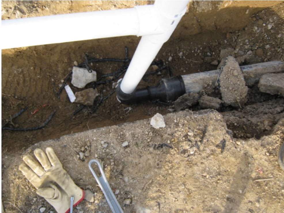
Photograph 3: Four-inch conveyance line with riser and "T"-fitting for aboveground connection to SVE well.
