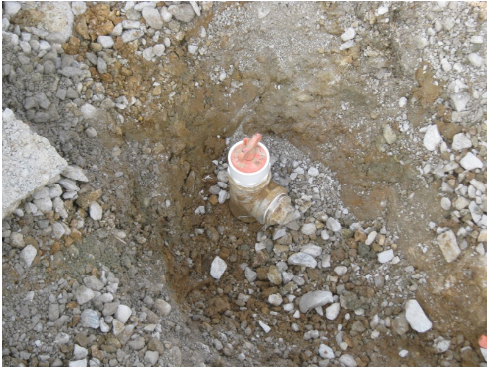
Photograph 1: Two-inch well head "T"-fitting with connection for conveyance line capped.
