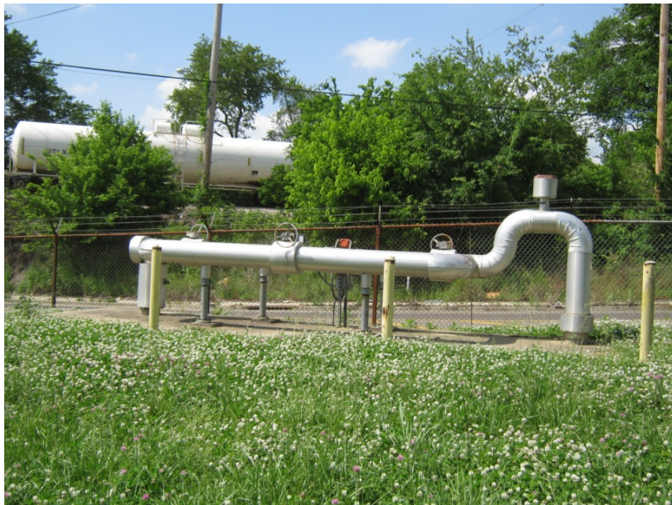
Photograph 6 – Sanitary Sewer Discharge Loop
