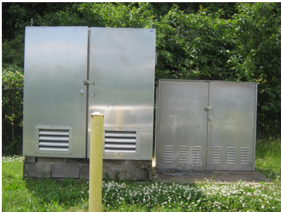
Photograph 3 – Recovery Well (RW) Enclosures
