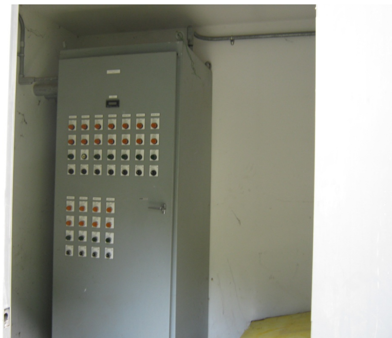
Photograph 2 – IRA Control Building Interior, Control Panel
