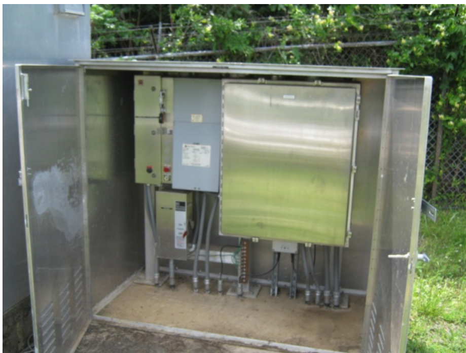
Photograph 4 – RW Control Enclosure
