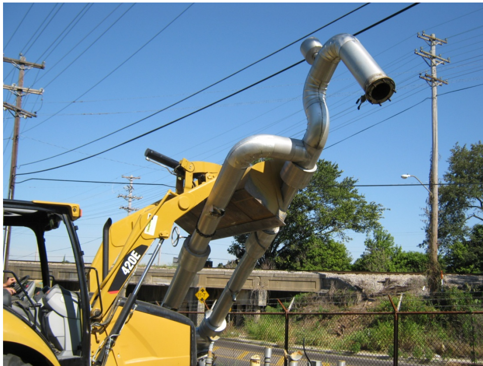
Photograph 10 - The discharge loop was removed from its pad.
