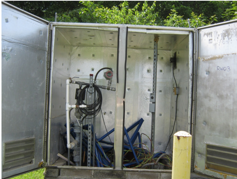
Photograph 5 – RW Pump House
