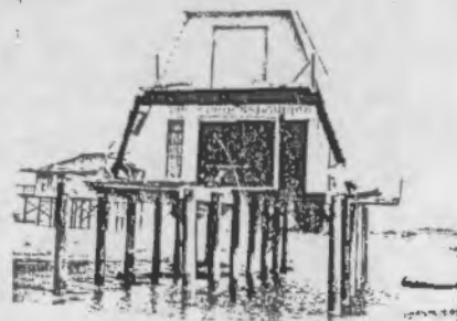
Fig. 14. Ground photo of damaged beach front home and the channel scoured underneath.
