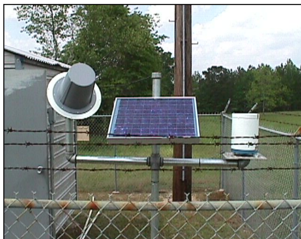
Figure 5-2. Typical Field Installation of a Precipitation Gage
